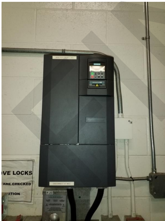
Figure 4. VFD with no protection
